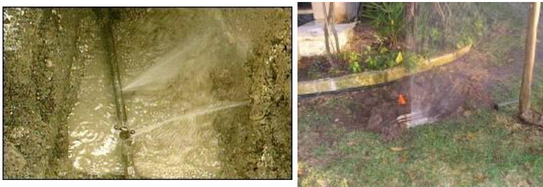
Figure A.6 – Service leak
