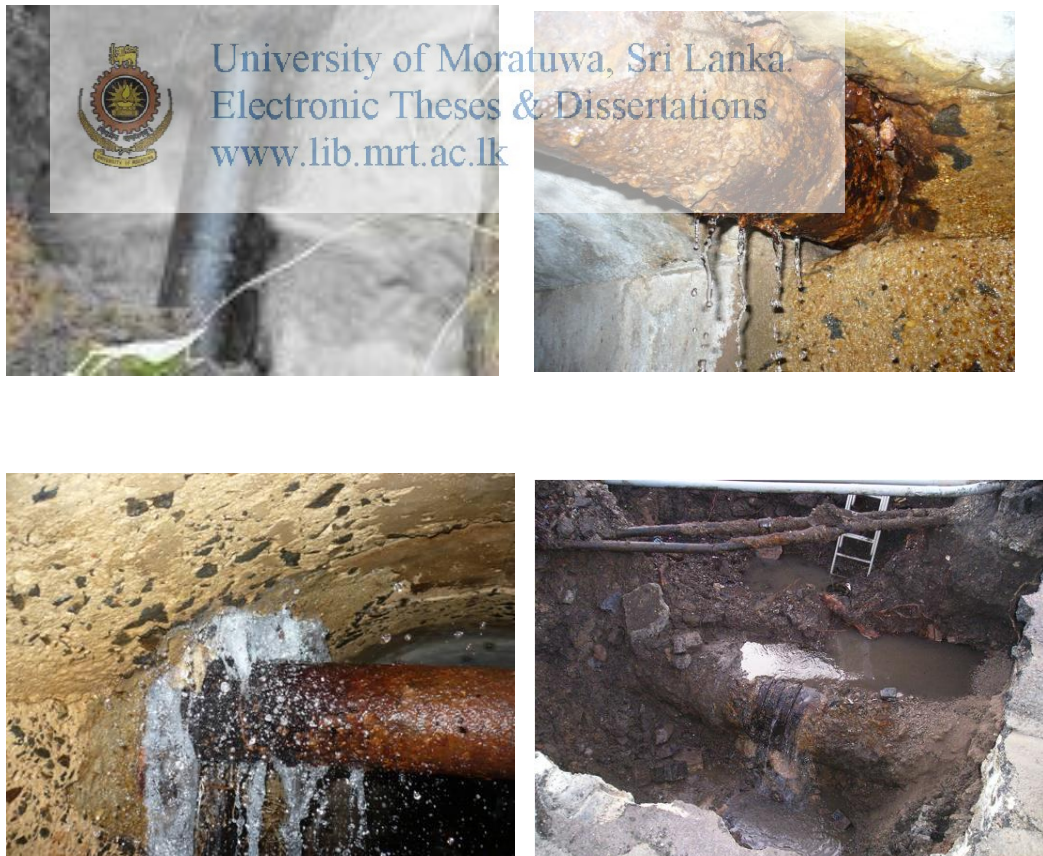
Figure A.5 – Major leaks
