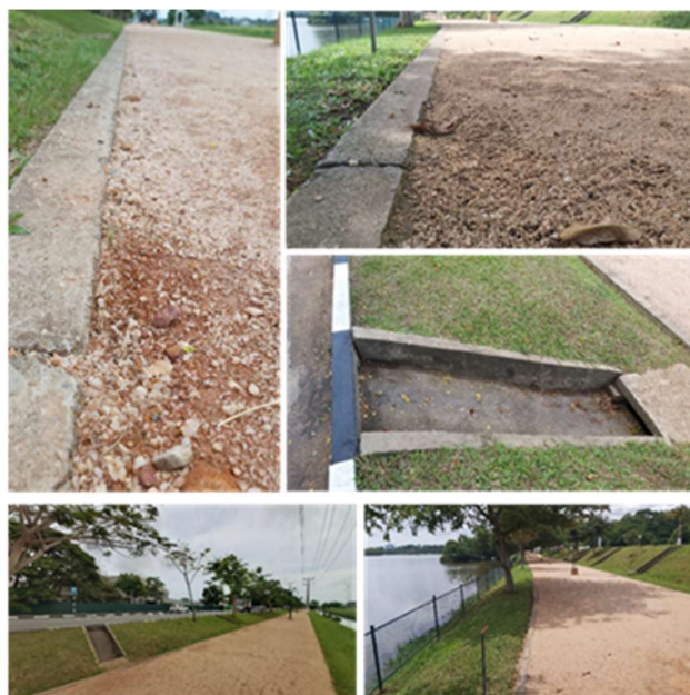
Figure 12: Drainage systems and the used raw materials for the jogging tracks Source: author
